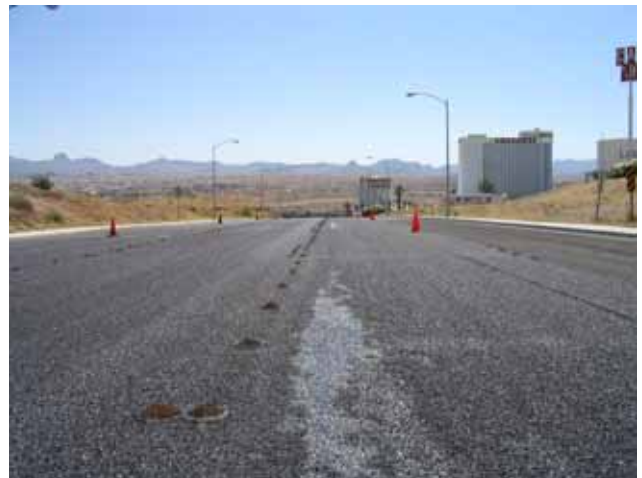
4. Raveled appearance of open grade mix. Civic Drive
